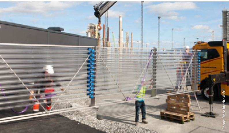
In the Silicon Valley of the Sea, which is currently under construction, the aim is to create an aquaculture with sustainable sources of feed by using photobioreactors.
