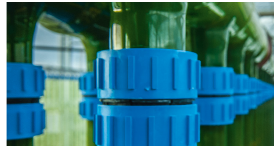
Manifolds and couplings, fence system. © Jongerius ecoduna GmbH
